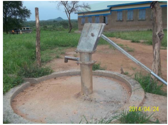
Broken down borehole in Kapoeta East School County
